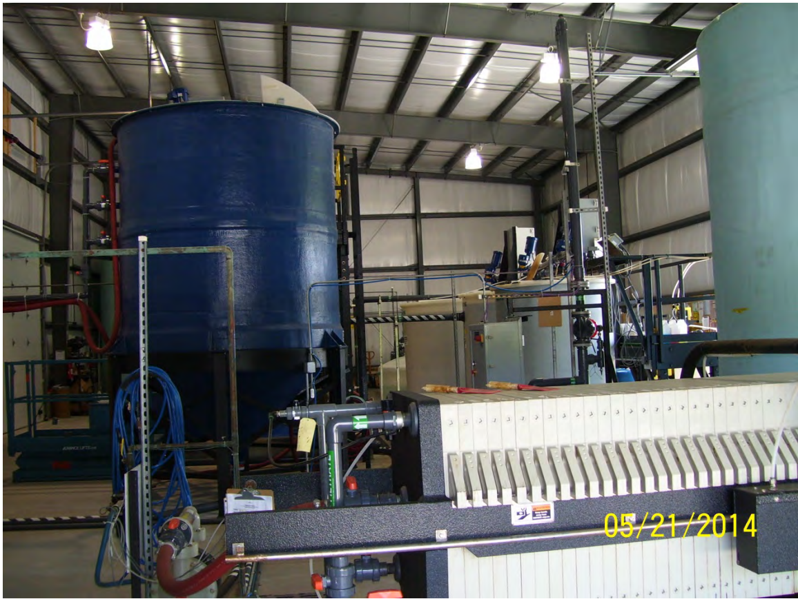
View inside groundwater treatment plant
