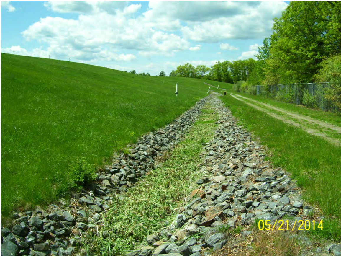
View of northern bottom-of-slope drainage channel showing standing water and vegetation
