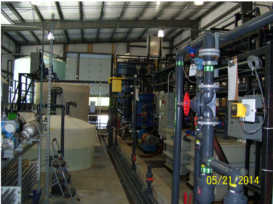
View inside groundwater treatment plant
