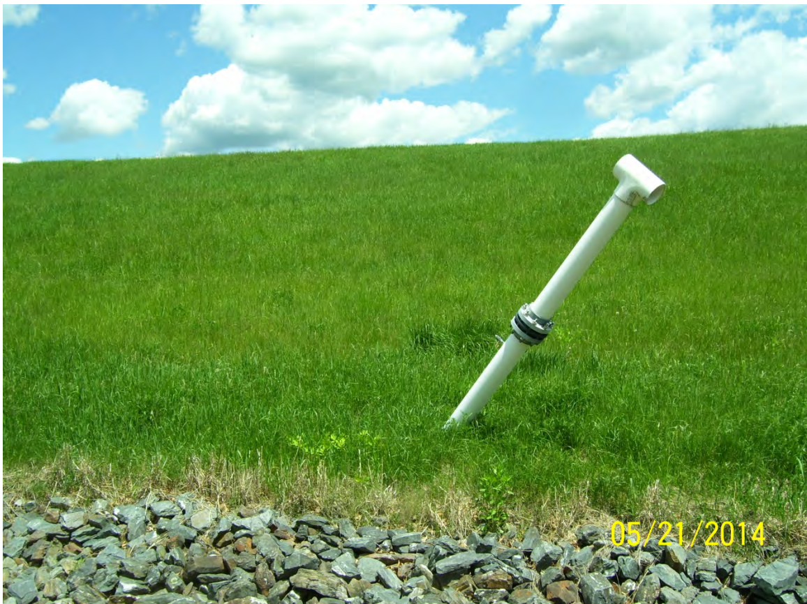
Tilted passive landfill gas vent in southwest area of landfill
