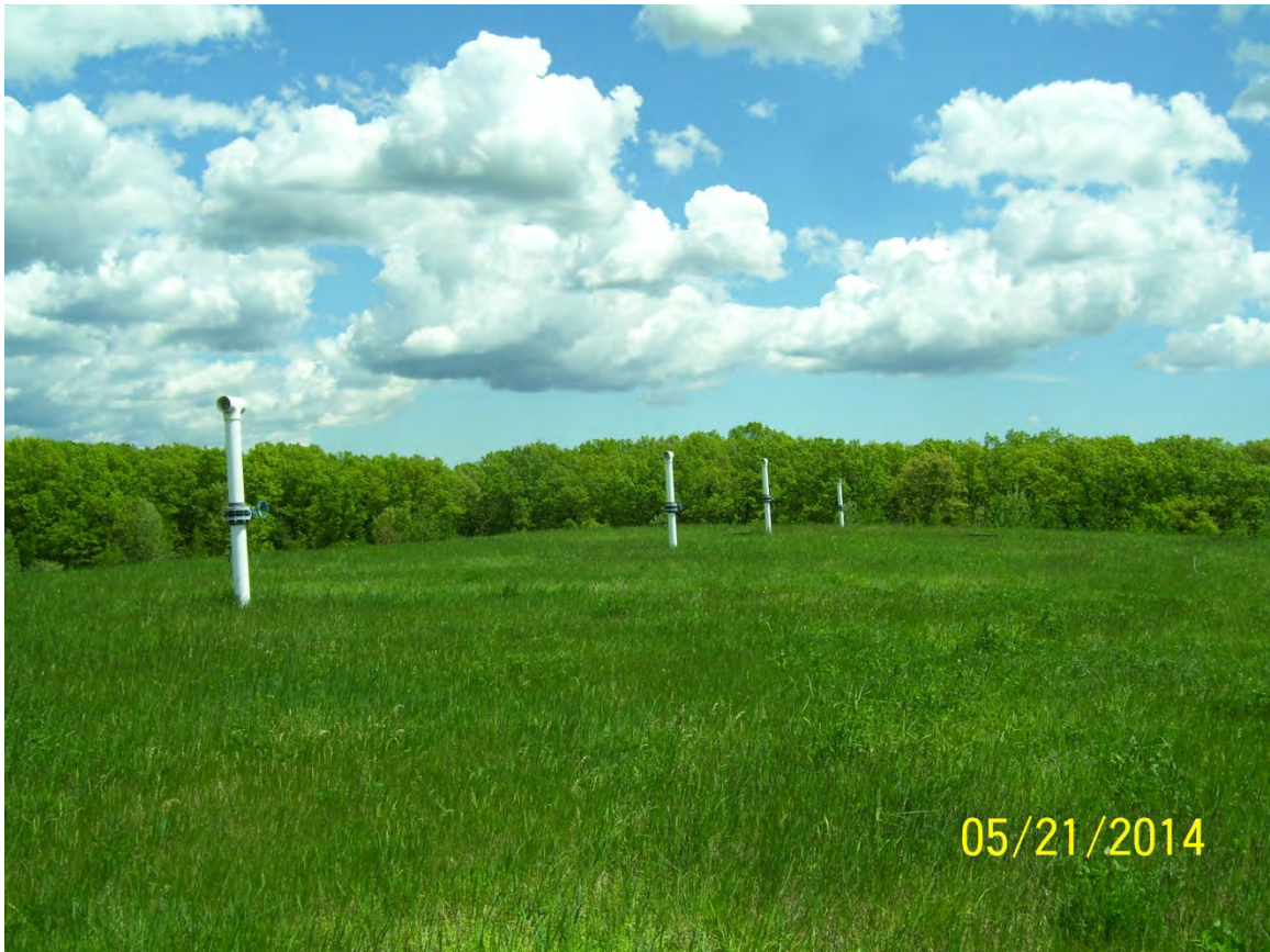
Passive gas vents on top of landfill, facing east
