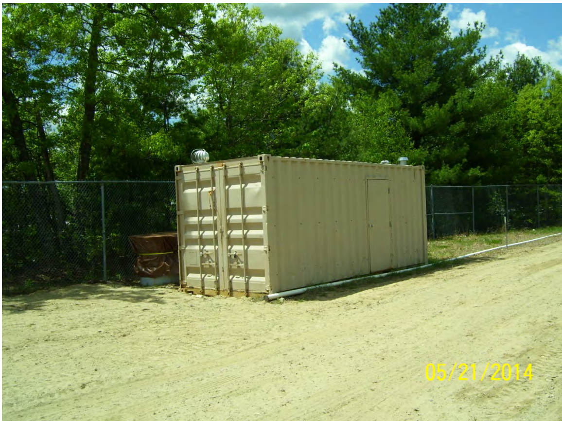
Groundwater equalization tank in southwest area of landfill
