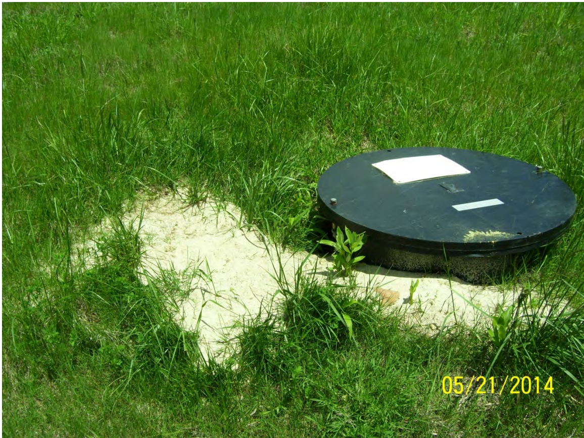
Animal burrow next to landfill gas monitoring point MP-4 on southern side of landfill
