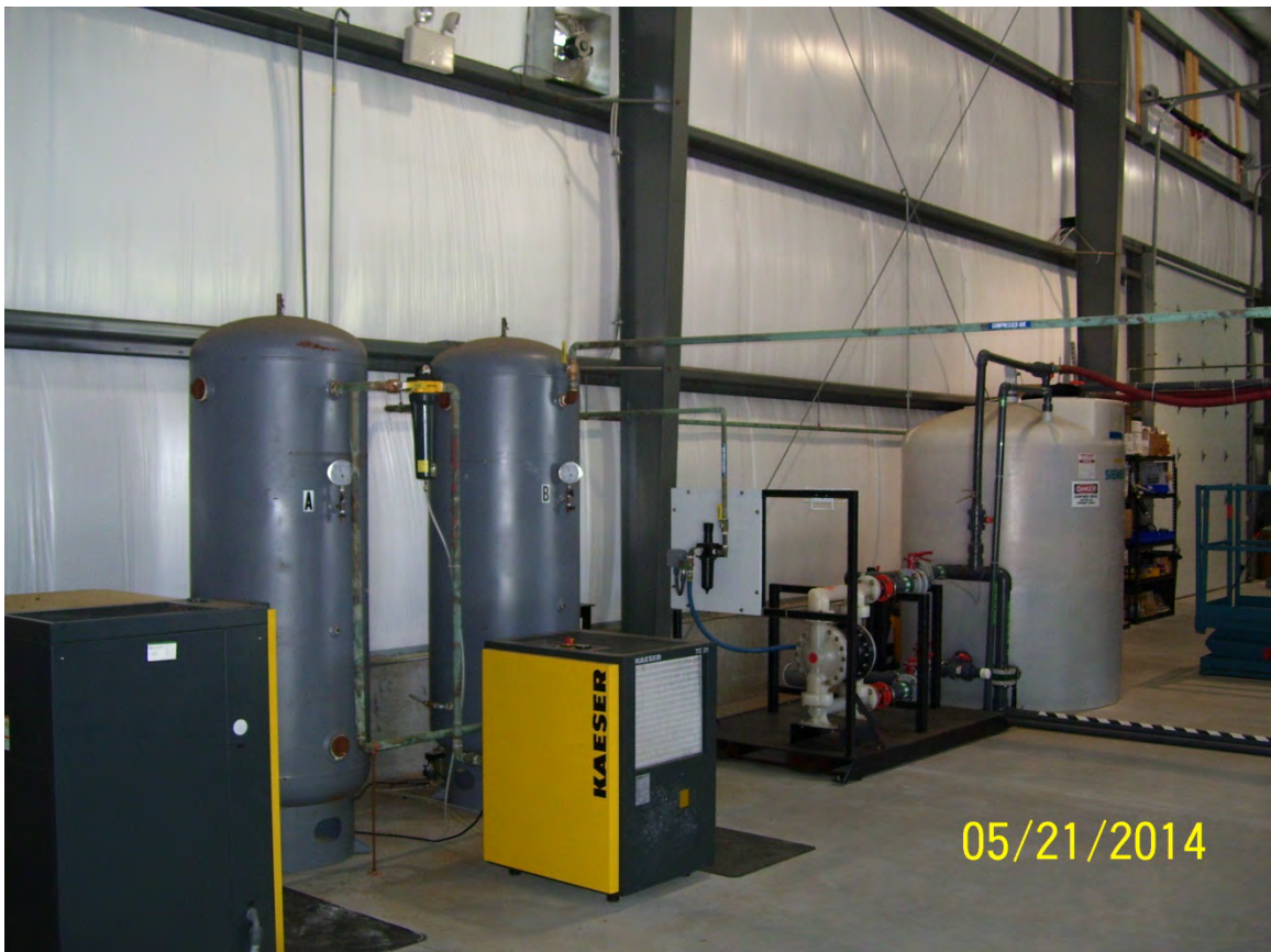
View inside groundwater treatment plant
