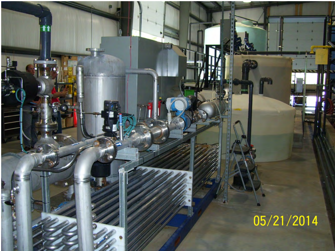
View inside groundwater treatment plant – Purifics unit
