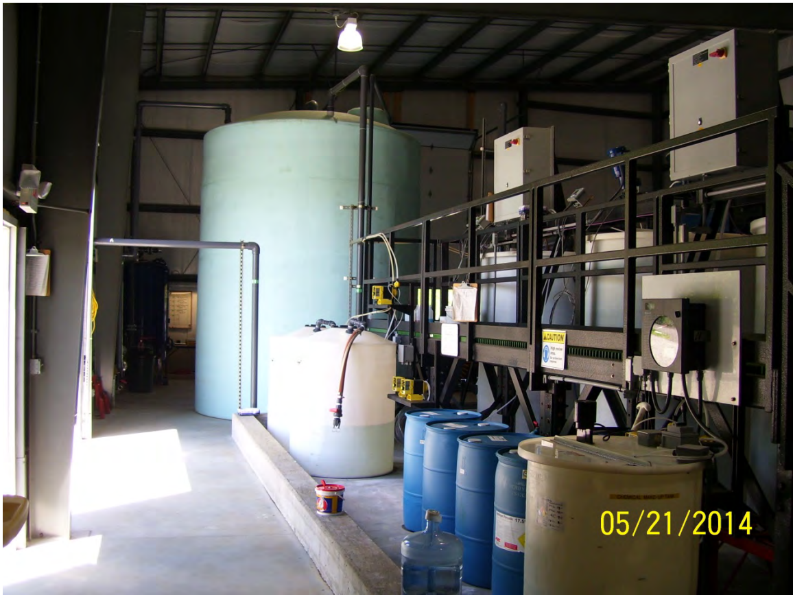
View inside groundwater treatment plant
