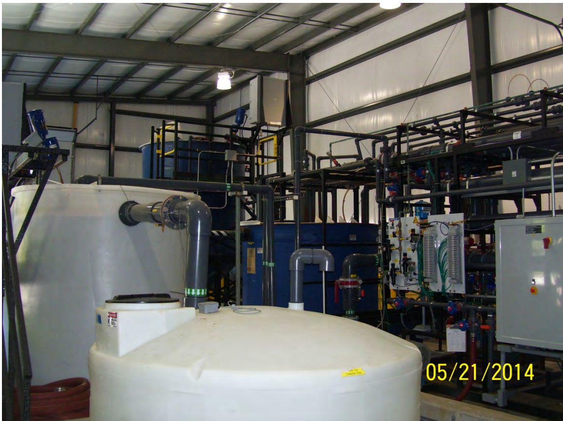
View inside groundwater treatment plant
